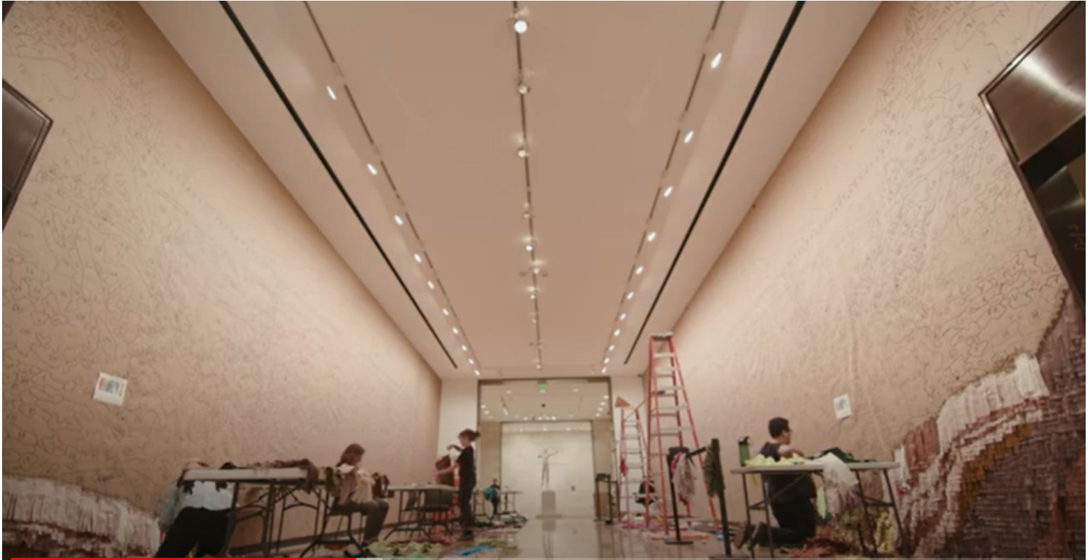
Figure 9. Process photo showing the paper covered wall, pattern layout, and beginning of installation process, from the short film The Making of Puente Nuevo , 2019.
