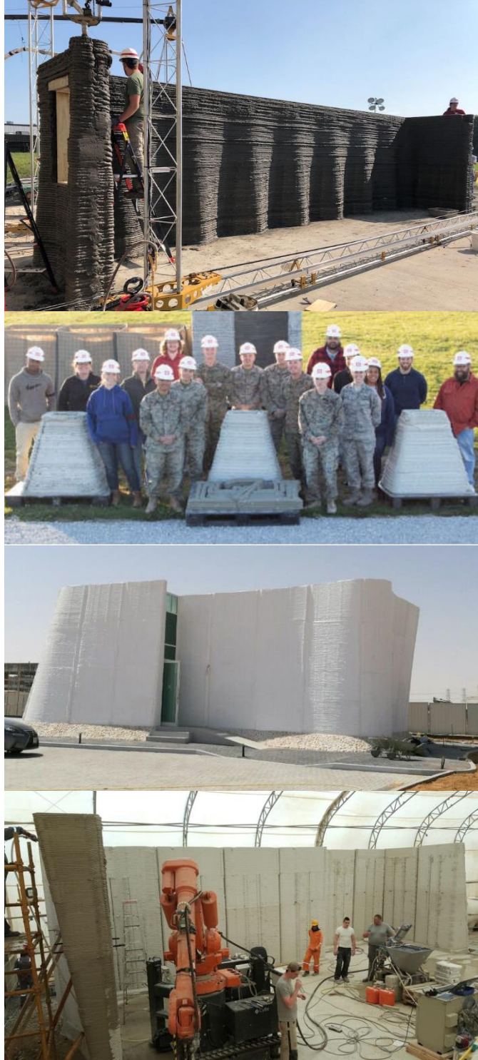
Figure 3.18 Examples of sloped surfaces in military experiments (precedent studies #8 and #9) with commercial example by CyBe Construction
