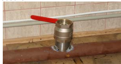
Figure 1 Basic assembly for connecting the intervention devices
