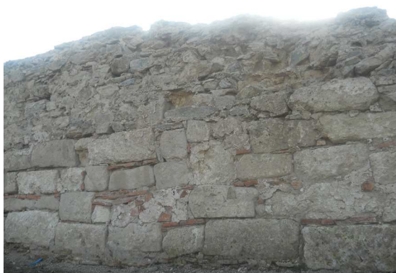
Fig. 28b Arched wall of the amphitheatre arena with visible repairs, details. Photo by the author.
