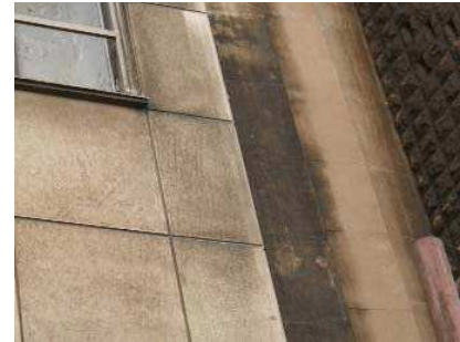
Figure 13 - Dirty wall surface of "Veselje" on building B
