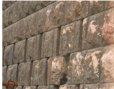
Figure 12 - Dirty wall surface of "Koral" on building B
