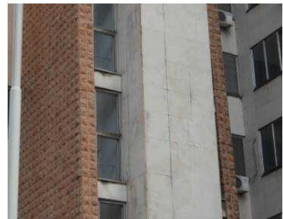
Figure 10 – Facade of the tower of the building B with stains on “Veselje” slabs
