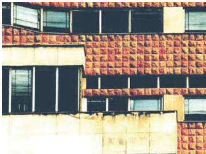
Figure 8 – Facade of building A with stains on “Veselje“ slabs
