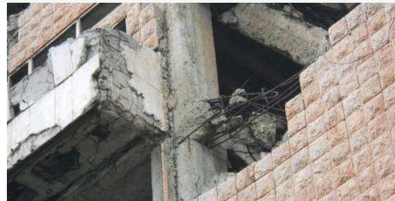
Figure 5 – Linear elements of construction with stone laid in cement mortar to the casted concrete
