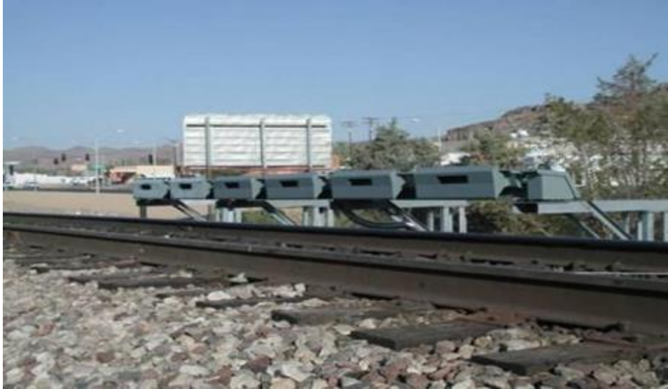
Figure 3: Trackside Acoustic Detector System (TADS™) [8]
