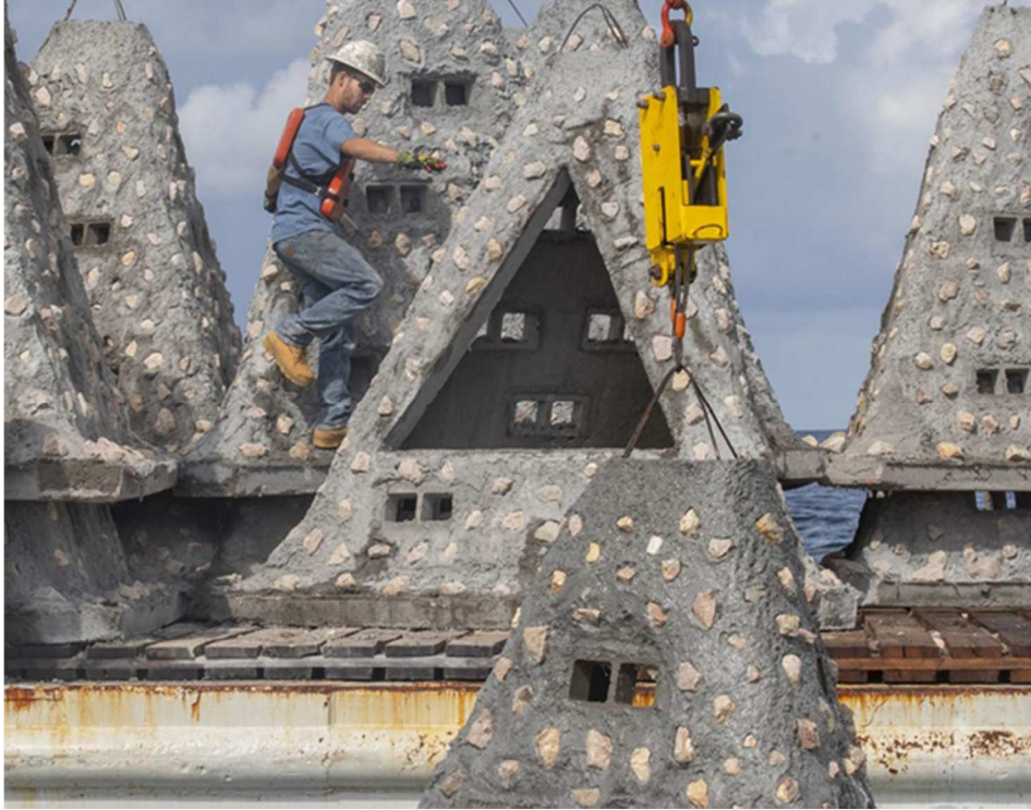
Figure 3: Concrete reefing pyramids used in the experimental reef area in the Rio Grande Valley artificial reef. ~3 m of vertical relief
