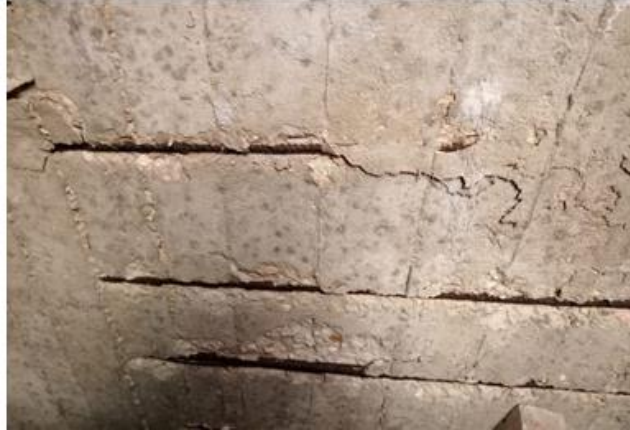
Fig.5: Corrosion of Steel Bars (Hulimka et al., 2020)
