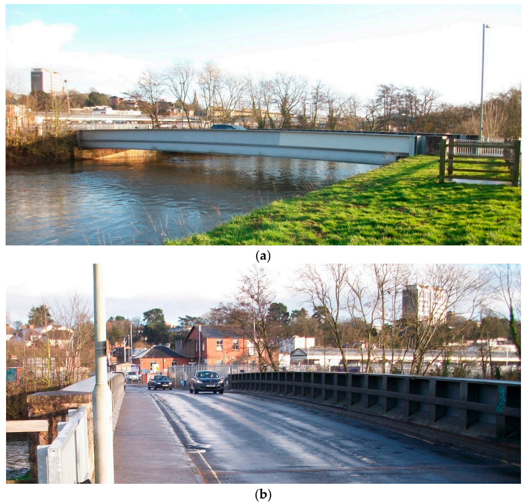
Figure 1. Bridge used in study: (a) north elevation; (b) bridge deck looking to the east.
