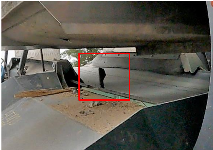
Figure 27. Main conveyor belt failure. The view is from the discharge area of the magnetic separator.
