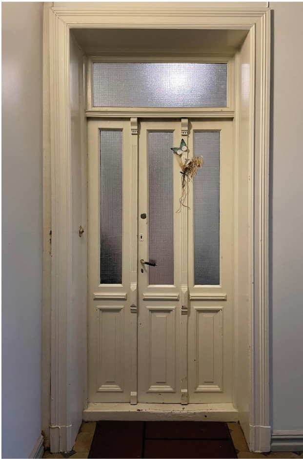
Figure 1. Typical stairwell door from a historic masonry residential building in Oslo, view from the stairwell side. In this example, the original glass panels have been replaced earlier with wired fire-resistant glass. Photo: Caroline Lundegaard Hannisdal, Murbyen, 2022.
