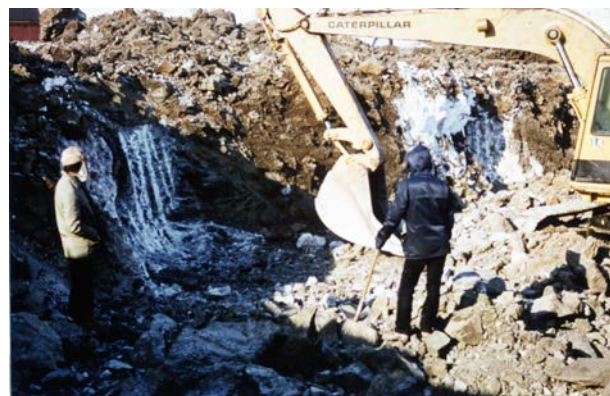
Fig. 7 Large ice-wedges in a foundation cavity on road 232. Normally traceable by ground inspection. Photo O. Gregersen
