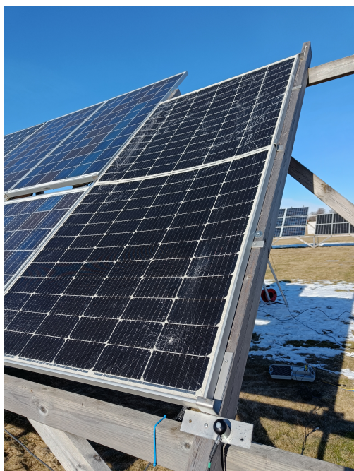
(a) Front side of the damaged module, PERC1.
