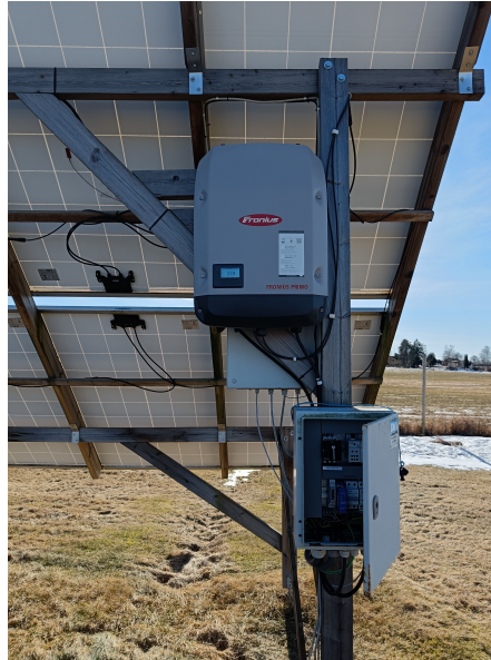
Figure 3.1.3: All modules used in the experiments are connected to a string inverter of the type Fronius Primo 3.0.
