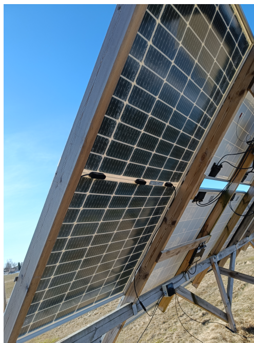
(b) Rear side of the damaged module, PERC1.
