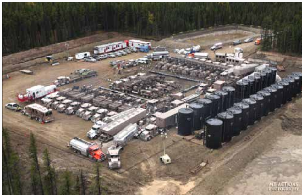
Figure 3.4 Hydraulic Fracturing Operation - Equipment and Layout
