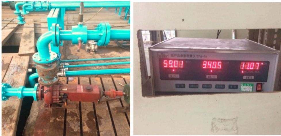
FIGURE 5 Pump performance test site.
