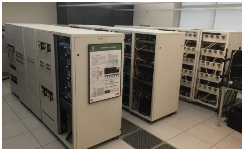
(a) Converter-based HTB cabinets
