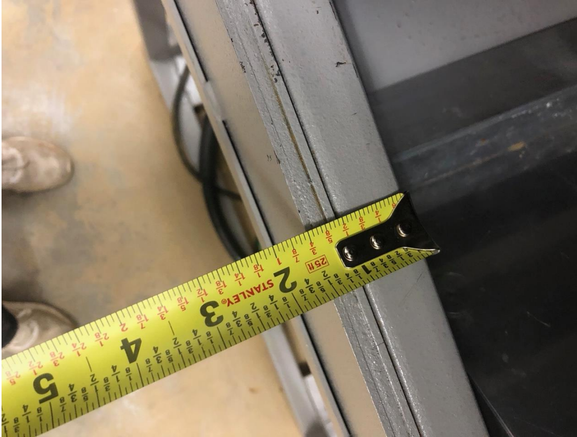
Figure 17. Measurement of the sandwiched lead shielding in the X-ray cabinet before modification. 1/8 in. of steel, 1/4 in. of lead, and another 1/8 inch of steel are shown. The 1 in. steel piece at the end of the tape measure is a structural steel tube.
