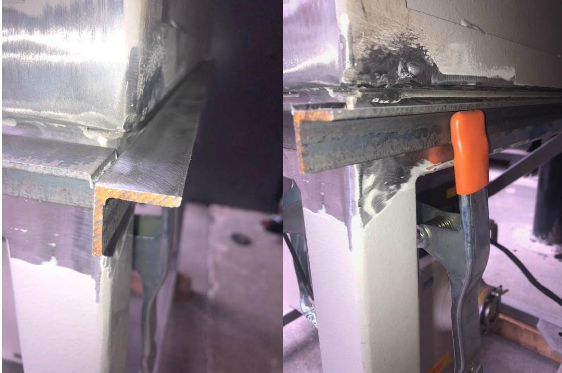
Figure 22. Image of 1 in. angle iron being fixtured with clamps on each face before welding.
