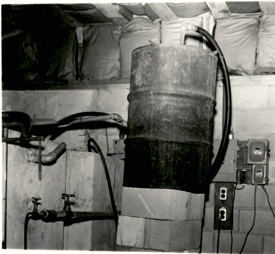
Figure 20. Mechanical Coagulant Mixer Showing Drum, Top Intake, and Side Discharge.
