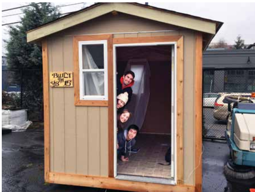
Sarah Brown, Chen Dong, Connor Leahy and Triet Tran from ME Team 17.5 take measurements of the Tiny House for the homeless for which they optimized the heating, lighting and ventilation systems.
