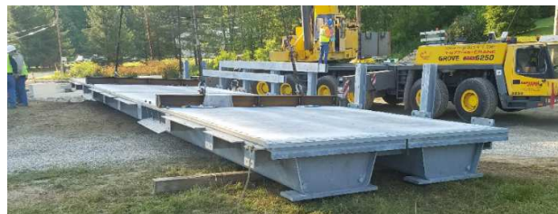
Figura 12: Módulo de construcción del Cannelville Road Bridge, (The Short Span Steel Bridge Alliance)
