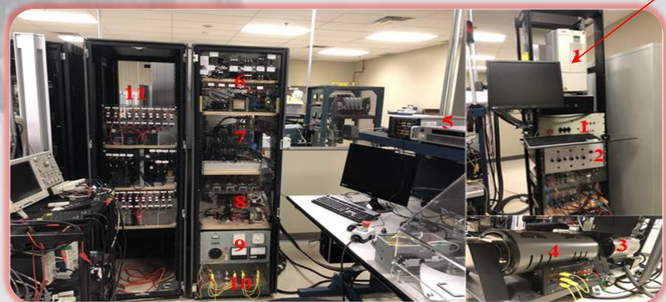
Benhalima, Seghir, Rezkallah Miloud, and Amrish Chandra. "Real-time implementation of robust control strategies based on sliding mode control for standalone microgrids supplying non-linear loads." Energies 11.10 (2018): 2590. Hardware Prototype
