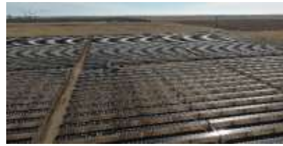
27.5MW Johnson Corner (KS) Power contract: Sunflower Electric
