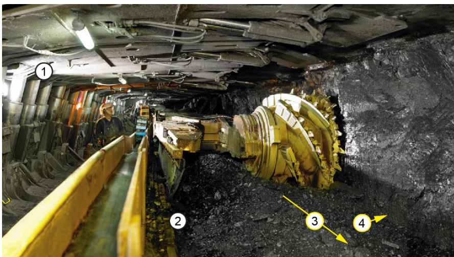
Figure A-3: Longwall shearer and armoured face conveyor operating at the Twentymile mine [225] 20
