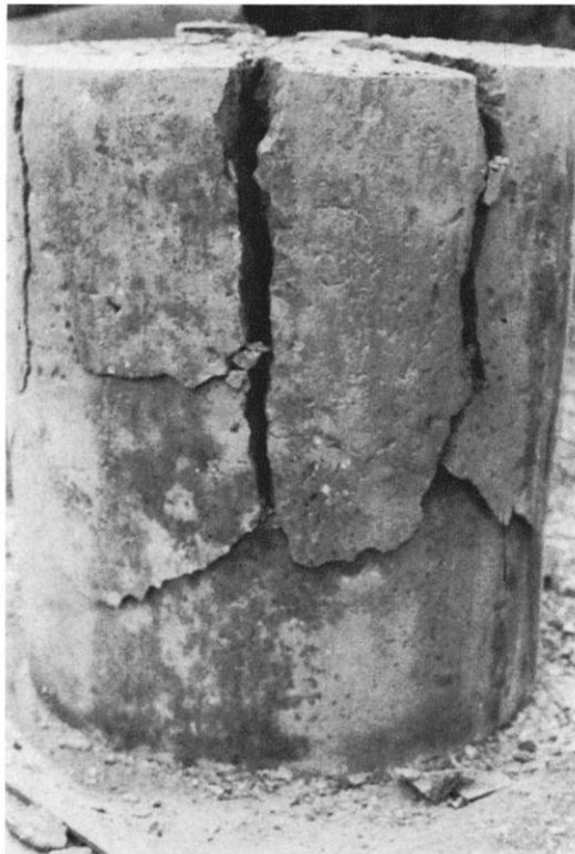
FIG. 15. Fractures in concrete.
