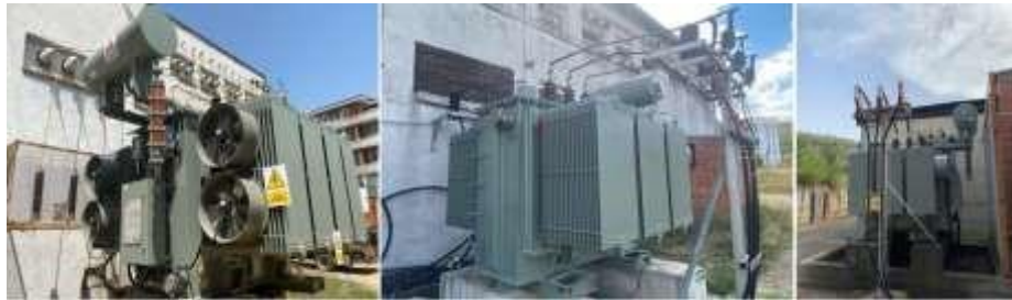
Fig 6 Power transformers in the distribution network, SS 35/10 kV “Xerxa”
