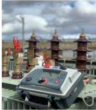
Fig.1. Insulation resistance measured directly with Megaohmmeter
