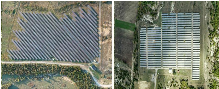
Figure 3. a) Eco Park, Madanaj- Kusar, Gjakove, 3,000 [kW] dhe b) Solar Green Energy, Novoselle, Kamenice, 3,000 [kW] [10]
