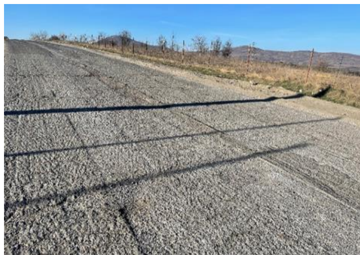
Figure 6. Asphalt erosion on the roads that will be replaced with the final 5 cm layer
