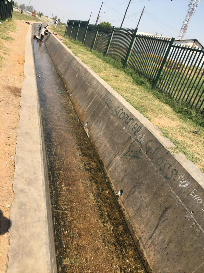
Bombay drainage system - social networks around washing and drawing water including playing area for children
