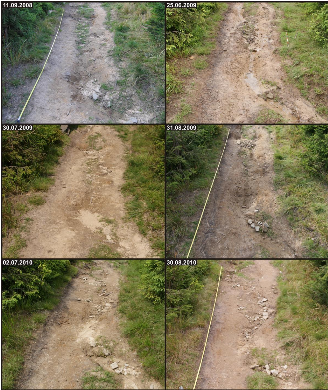
Fig. 4. The state of the trail and its surroundings for the selected dates – test field (P)ZLOMISTY. Notice the small plunge pools filled in with material and subsequently eroded
