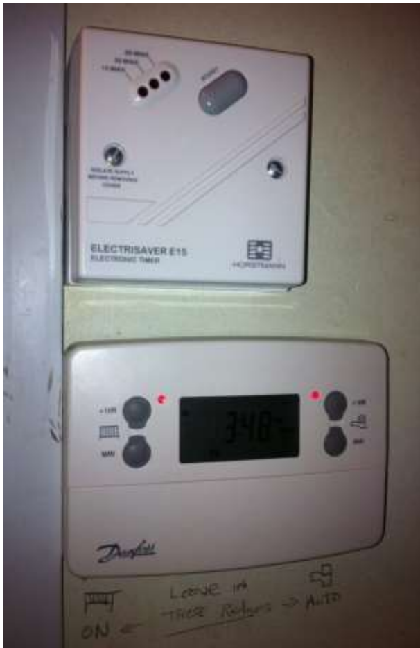
Figure 1(a). Hot water boost (top) and main control with handwritten instruction to leave in set positions (below).
