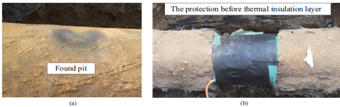
Fig. 6. (a) The found pit based on the data difference extraction result and (b) the protection for the pit area before the thermal insulation layer.
