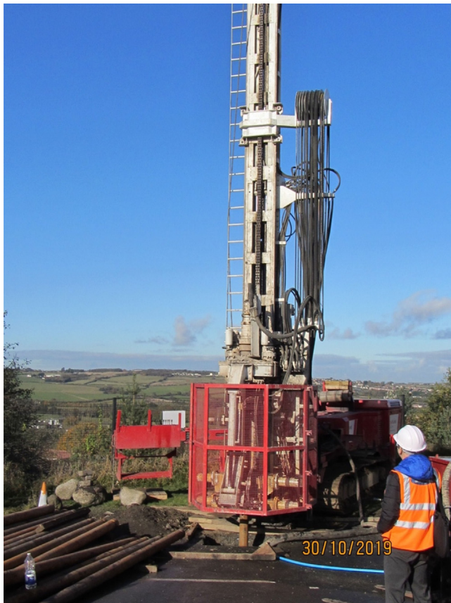
Fig. 4. Drilling at the Louisa Centre, Stanley, County Durham (October 2019). The well drilled into the former workings of the Louisa Mine from which water will be pumped to heat the adjacent swimming pool. The modest scale of the operation which is the size of a couple of parking spaces in the Louisa Centre's car park is clear from the photograph (photograph S. McDonald).
