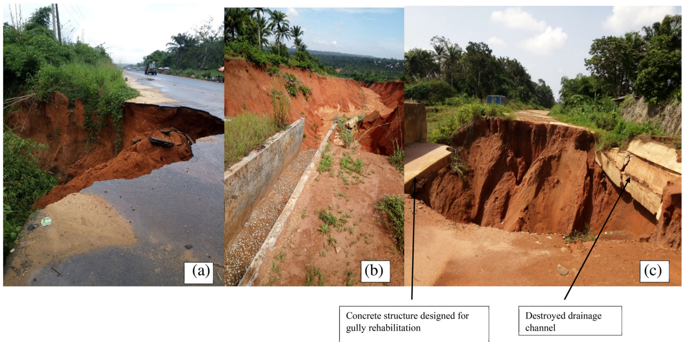
FIGURE 4 Proximity of gully heads to main roads. (a) Shows a moving truck close to a gully in Okwudor, Njaba LGA. In the first month of fieldwork (April 2019), no gully was identified on this axis of the road, but in June when the picture was taken, it had grown to where it is now in the picture. (b) Shows drainage structure which empties into a newly formed gully in Obibi-Ochasi, Orlu LGA. Road construction was abandoned at this site and eyewitness account suggests that (b) started in 2017 following abandoned road construction. (c) Shows gully head advancement following abandoned gully restoration project in Umueshi community. The gully destroyed the local road connecting two communities. Also visible in (c) are destroyed drainage channels which deliver runoff directly into the gully and concrete structure designed to control gully erosion [Color figure can be viewed at wileyonlinelibrary.com ]
