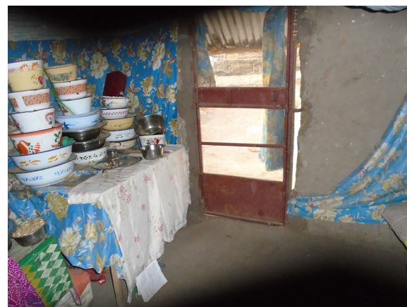
Fig. 11 PV poorly installed RooPfs backdoor
