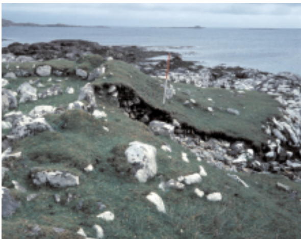
Figure 8.11. Site L7, a blackhouse on the east coast of Barra. The southern wall has been breached by the scouring effect of the tide.
