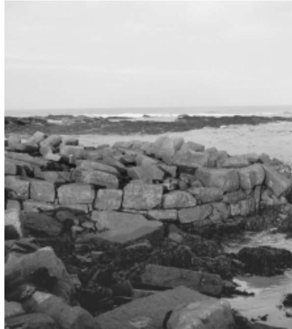
Figure 12.8. Footings of the collapsed north west pier of Kingsbarns Harbour.
