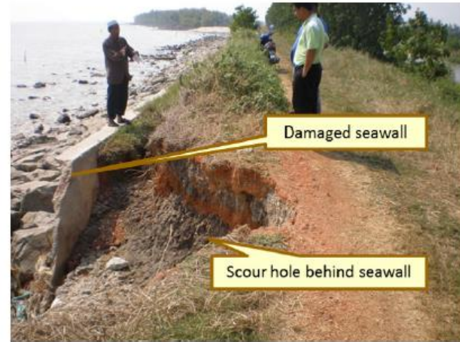
b) Seawall damaged after wave attacks (2010)
