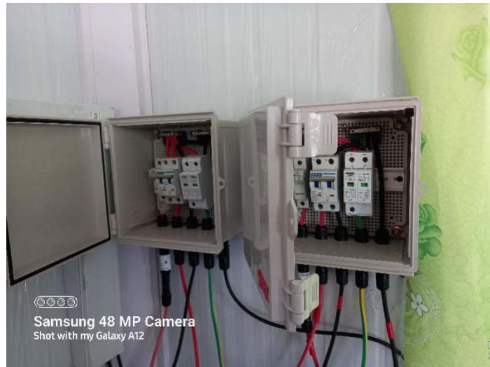
Gambarajah 10: Array Junction Box
