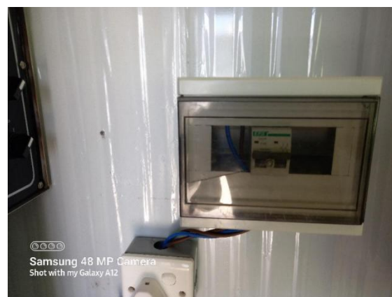
Gambarajah 12: AC Distribution Box
