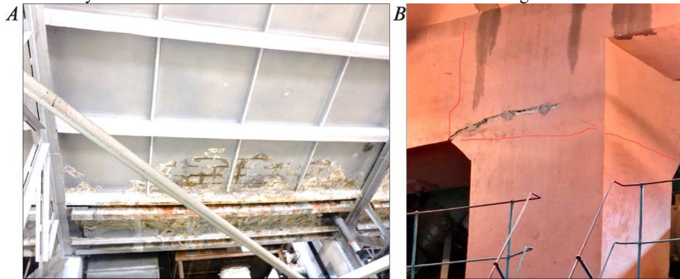
Fig. 2. A - condition of reinforced concrete slabs of the roof of the turbine hall and drainage gutter slabs. B - crack in the structures of the turbine generator foundation at the place of binding the supporting columns with the reinforcing belt.
