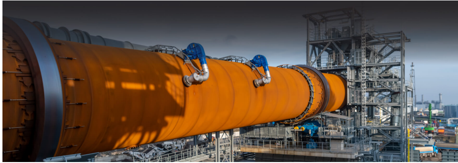
Figure 35: Rotary furnace used for the recycling of tar-containing asphalt, adopted from [28]
