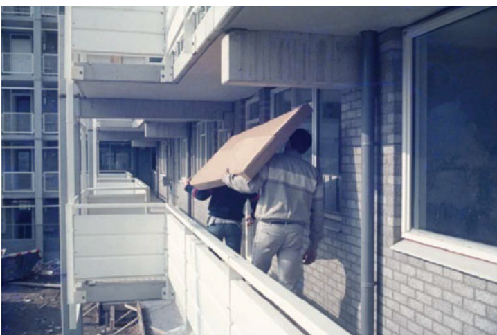
transport of the infill walls and making the bathroom with raised floor
