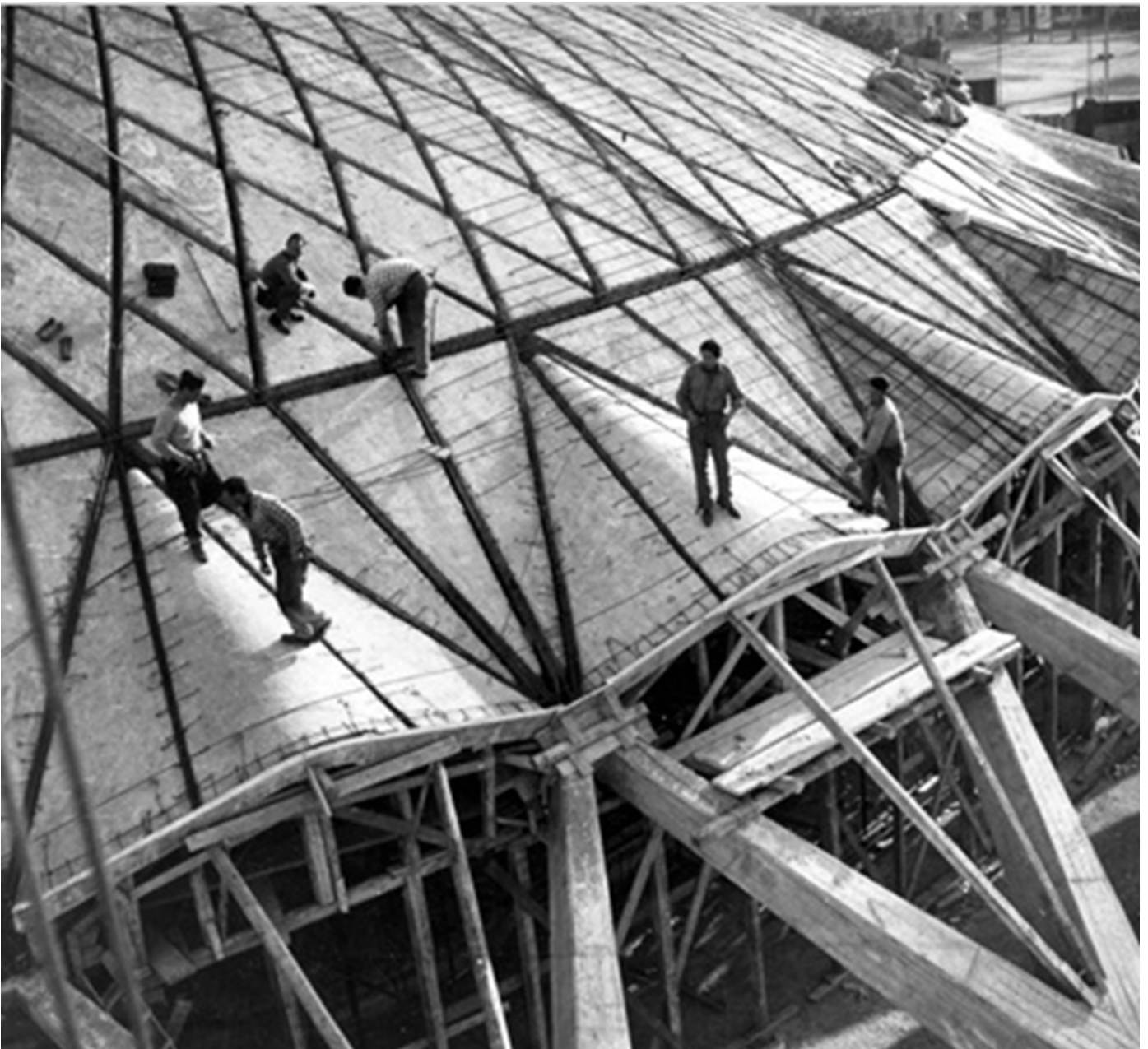
Figure 9 (Zoe Henderson, 2014) The assembly of the dome roof structure of the Palazzetto dello Sport
