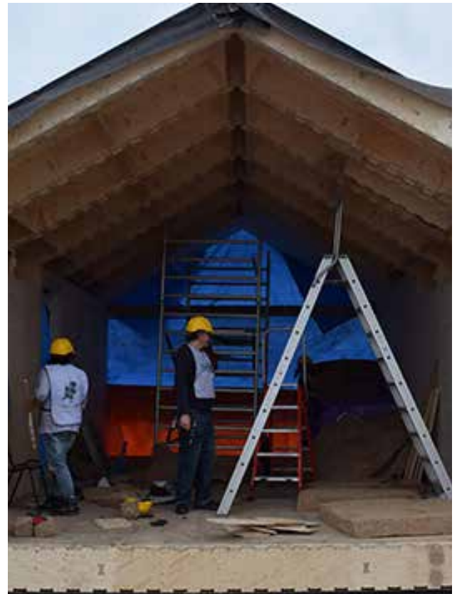
A.8 A WikiHouse with cladding and infill under construction (Woningbouw atelier, n.d.)
