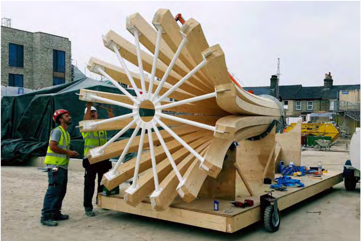
29. Timber structure element of Cambridge Mosque ready for transport (Blumer Lehmann AG, n.d.)
