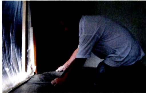
Figure 1.2: A non-ergonomic position can be seen when a tiler places a tile.
