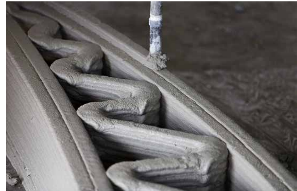
Figure 2.07 Supporting structure adjacent to the outer layers to improve buildability (CyBe Construction, 2019)
