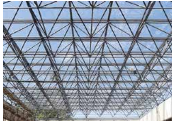
Image 71: Space frame in Station Almere centrum
