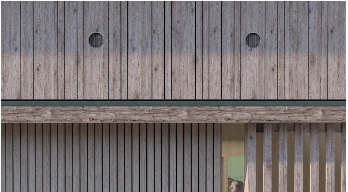
Figure 78: Ventilation shafts in façade for constant ventilation of the barn
