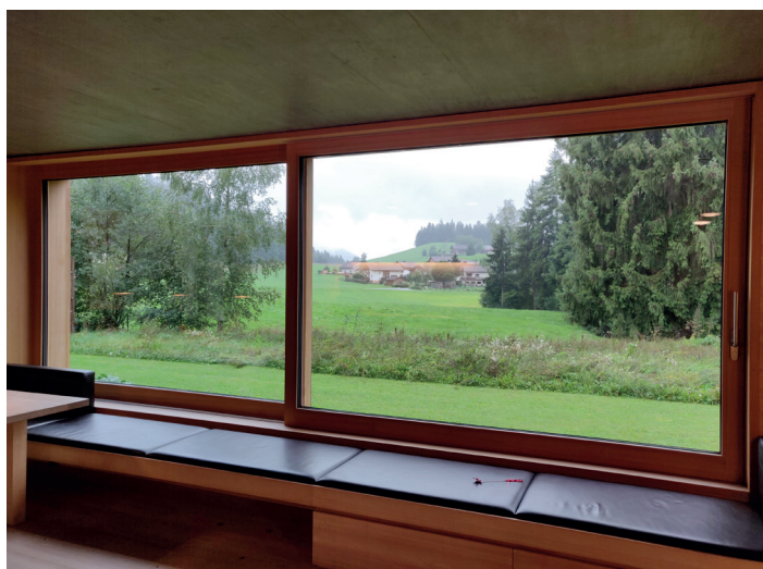
Figure 46: Window with insect screen located in the wall
