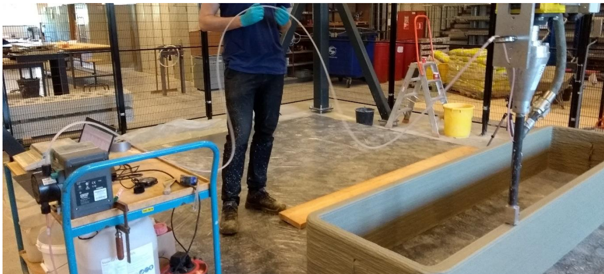
Figure 3-7 Liquid additive injection device. Left: schematic drawing. Right: detail image. Bottom: overview image of accelerator injection during printing.
