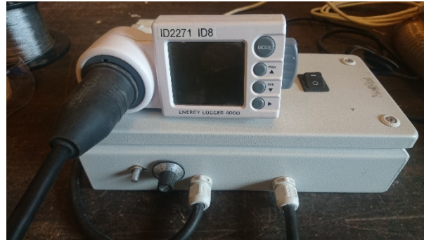
Figure B.10: Wattage meter in order to check settings blower.
