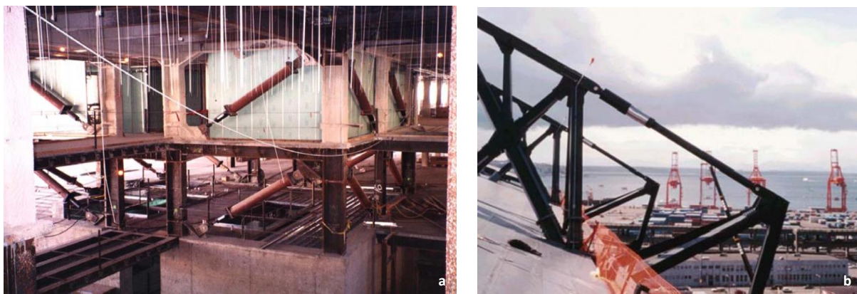
Figure 3.4: Seismic dampers in the San Francisco Civic Centre (a) and damping in the Pacific Northwest Baseball Stadium in Oregon (b)
