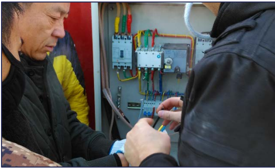
Figure 137; Connecting the Mobile factory to the electricity grid
