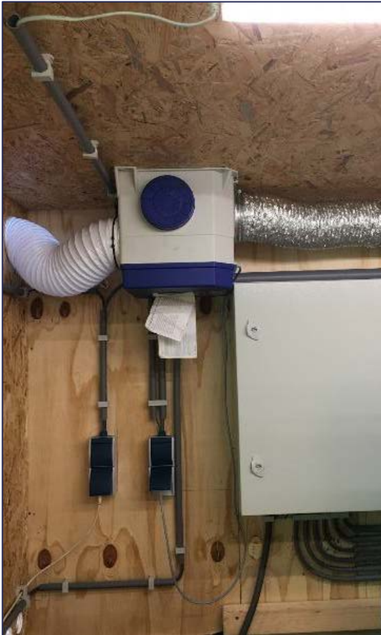
Figure 107; Vventilation unit of mobile factory
