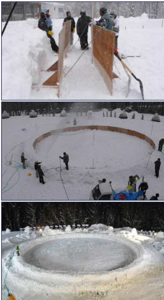
Figures 24-26; Building an ice ring with the use of a wooden frame work; source: (Kokawa, et al., 2012)
