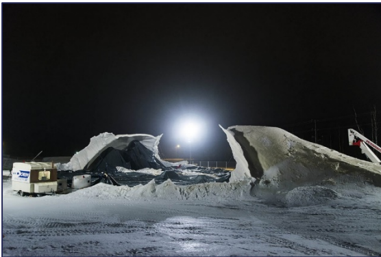
Figure 8; Collapsed bridge during construction; source: (Koekkoek, et al., 2016)
