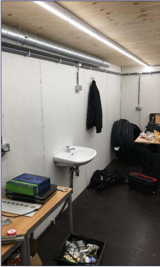
Figure 104; Electric sockets are connected as engineered in the electric circuit
