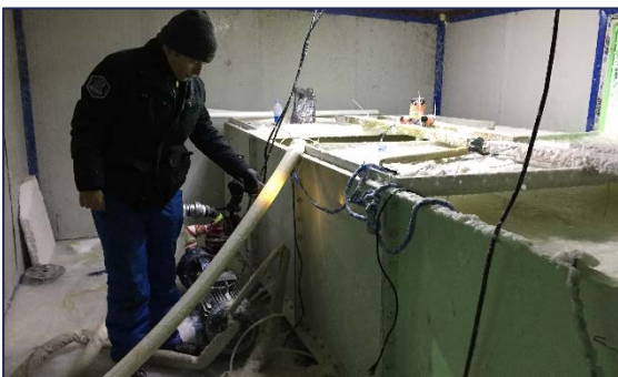
Figure 139; The improvised heated buffer room with a buffer capacity of 9 m 3
