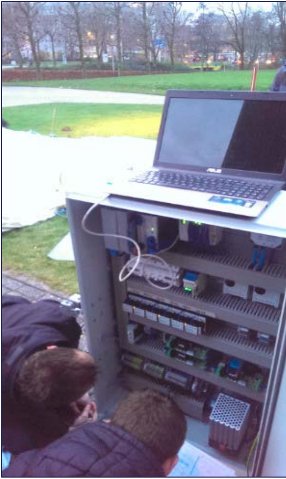
Figure 110; Testing of monitoring system
