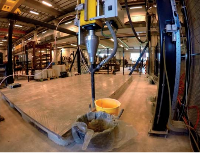
fig.1.3 Preparation concrete printer in the lab. Checking the amount of concrete coming out of the nozzle and its speed.
