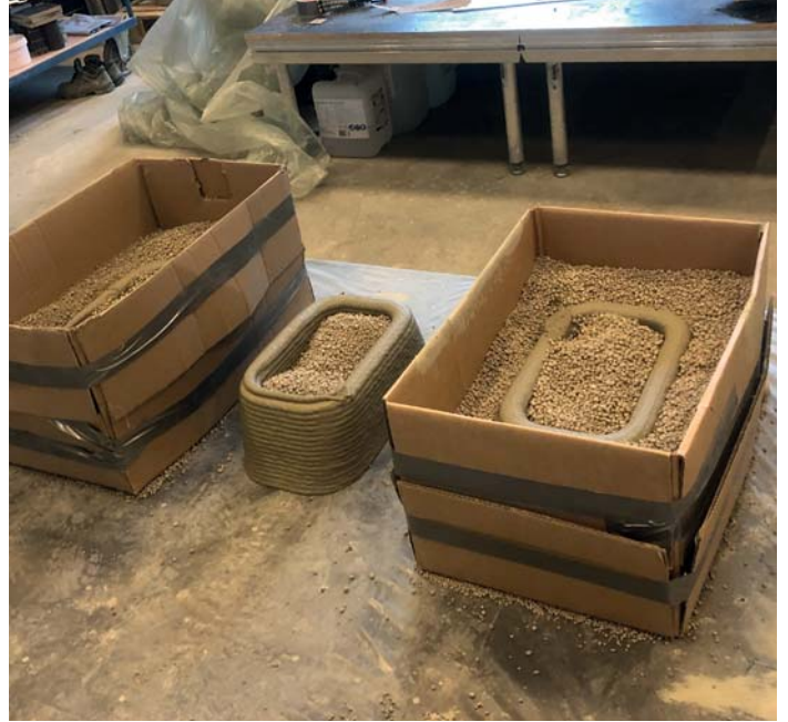
fig.1.7 Bookshelves for the Helix tower are printed - after having printed it, it is time to let it dry in the box with the filling material on the inside. When the concrete has become dry and hard, the box can be taken out and cleaned.
