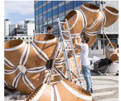
Figure 3.12. Assembly of the ICD/ITKE 2015 research pavilion which uses units that are in closed equilibrium (Bechert et al. , 2016).
