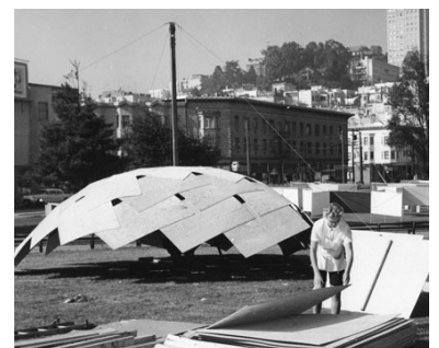
Figure I.4. With the addition of every plywood sheet, the final shape is further approached.
